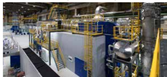
Alfa Laval Test & Training Centre in Aalborg
